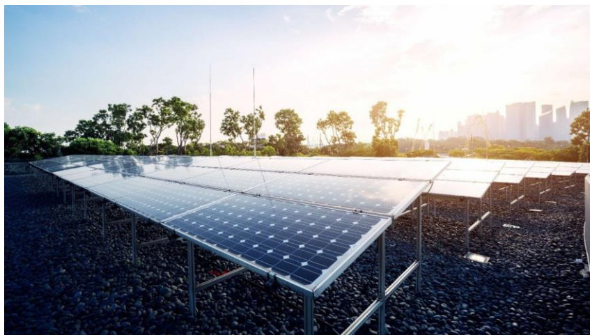
Figure 8.2: Rooftop Solar Panels
